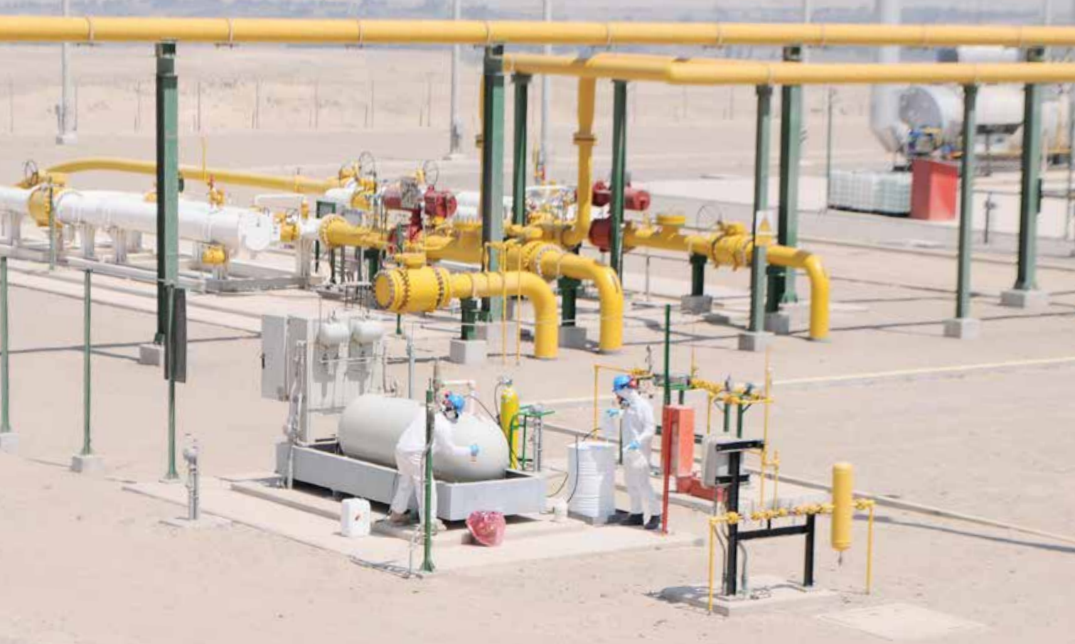
Contugas gas pipelines, Peru
