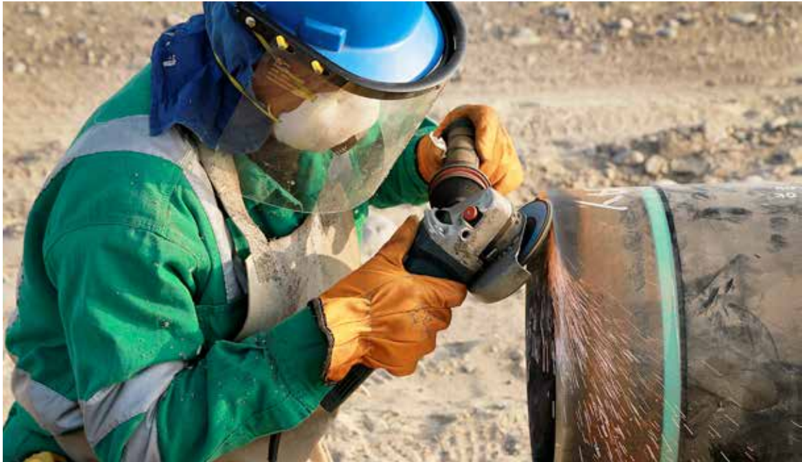
Use of adequate personal protection equipment is part of the GEB culture.
