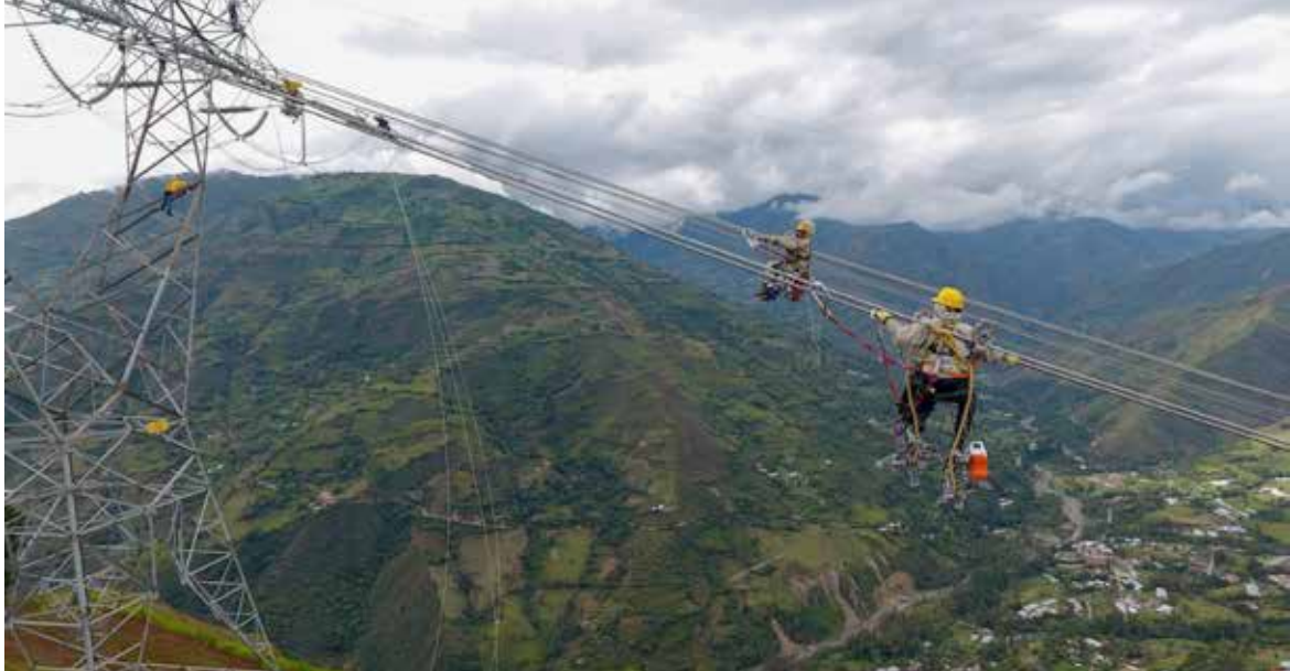
GEB transmission networks, Colombia.
